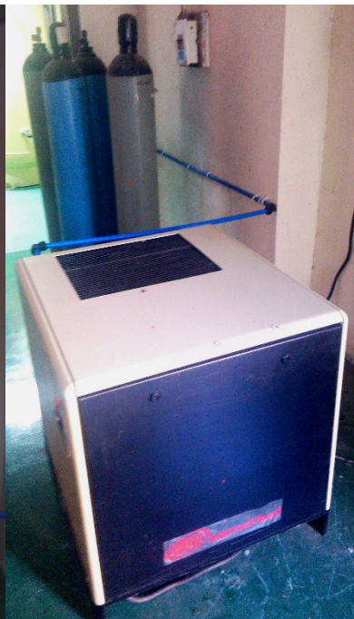
(c) Air Compressor System and Gas Cylinders
