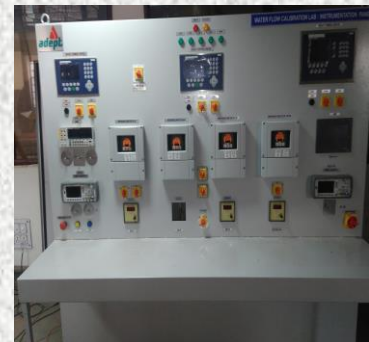
Instrumentation Panel of WFCF being upgraded
